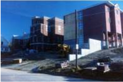
▲ The new facility was constructed directly in front of the old St. Joe's Home. Residents resided in the old facility until construction was complete.
